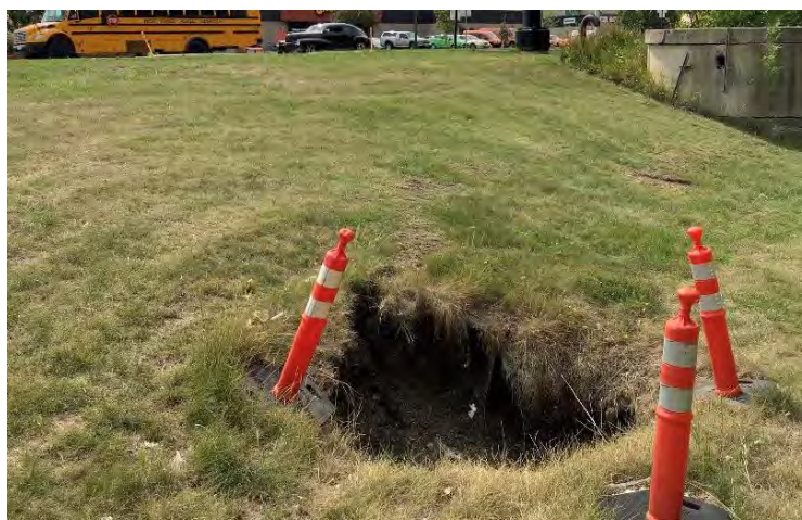
Figure 6: Sink Hole from Separated RCP Storm Sewer Joint
